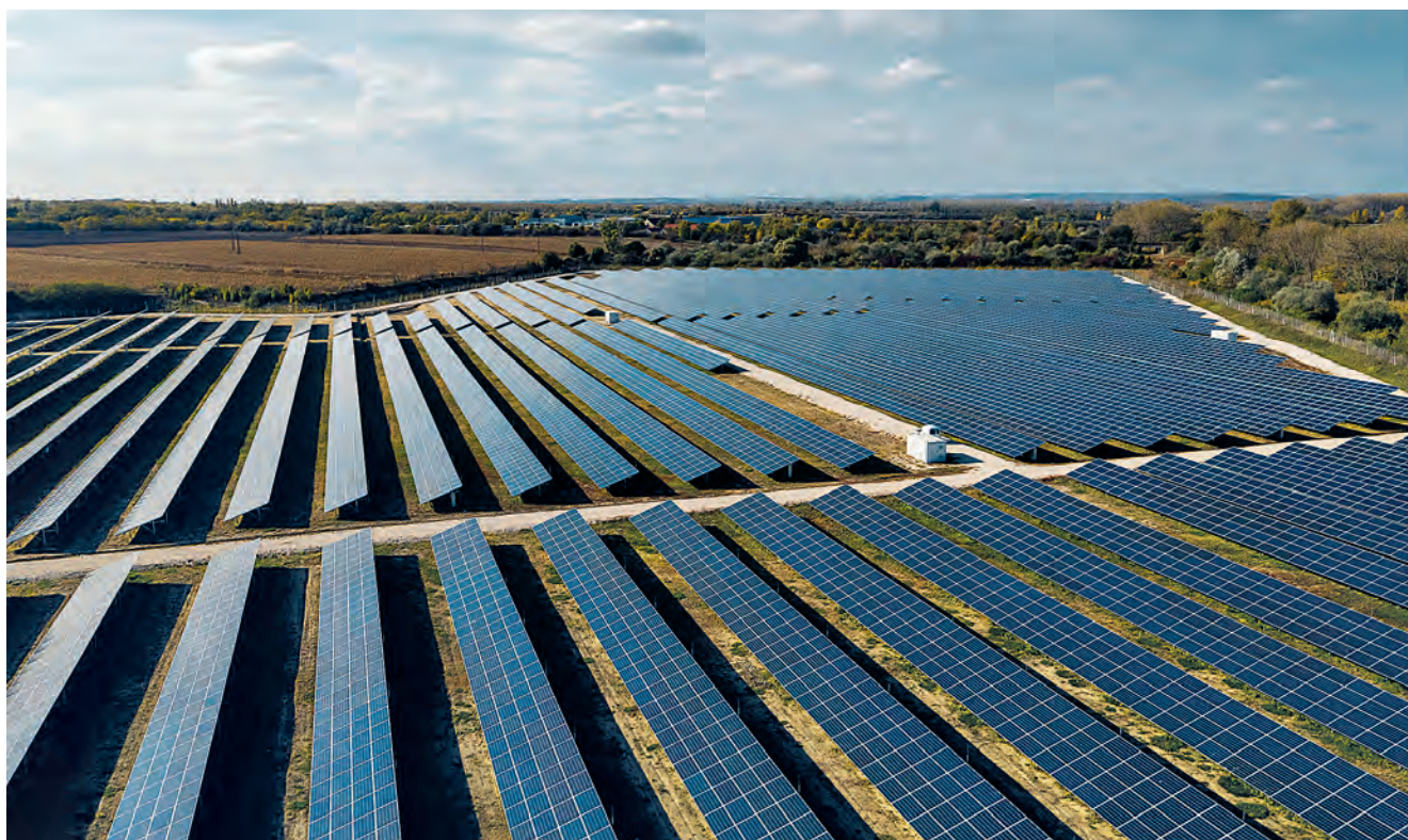
Keppel has grown its renewable energy portfolio from 3.8 GW as at end-2024 to 4.7 GW, including battery energy storage systems and projects under development, as at end-2025.
