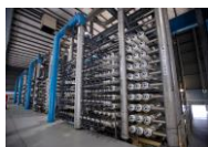
SingSpring Desalination Plant
