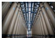
Keppel Seghers Ulu Pandan NEWater Plant
