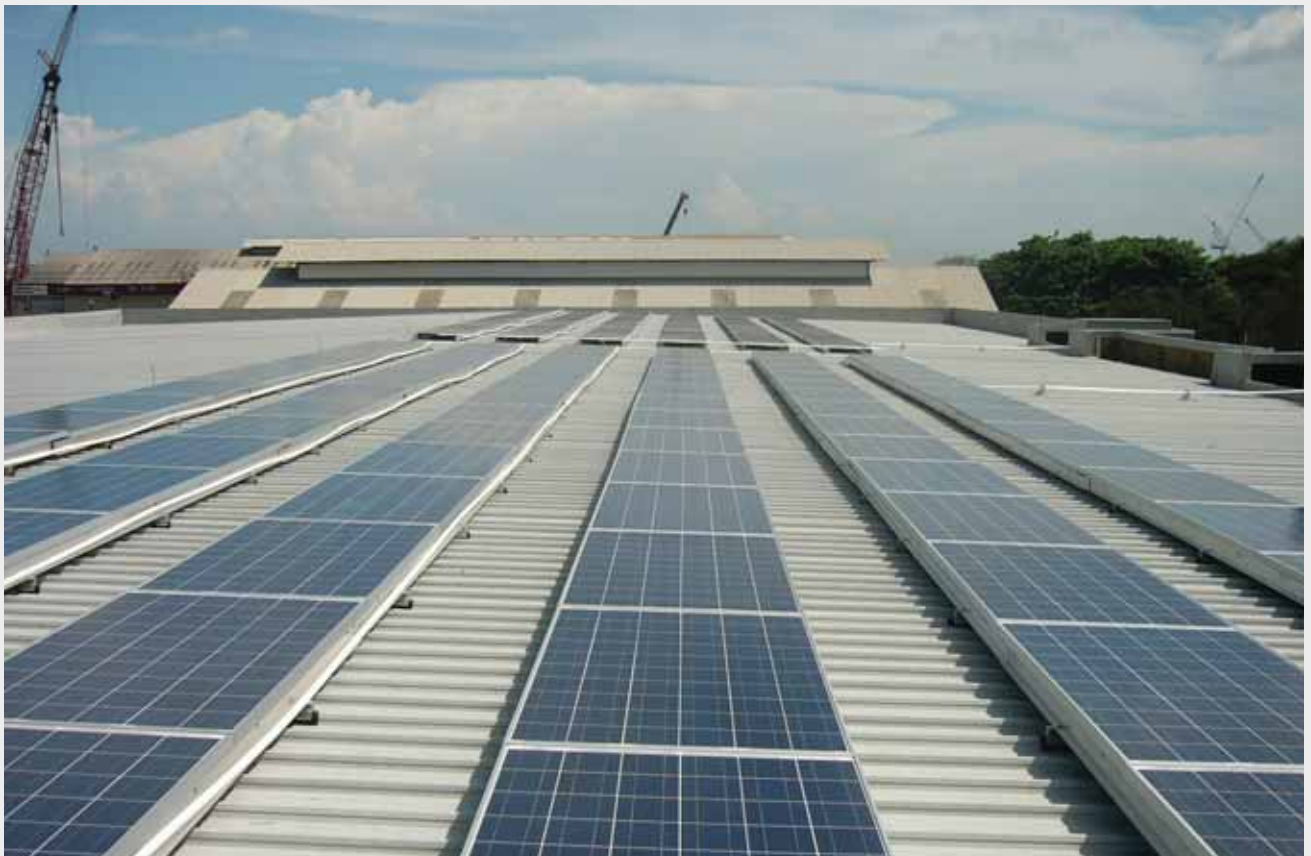
Keppel Offshore & Marine Technology Centre installed solar panels which potentially save up to 1.5m kWh annually.
