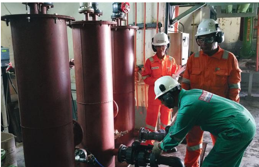
The Senoko WTE Plant effluent filtration system reduces the amount of NEWater consumed at the plant during dry spells.
