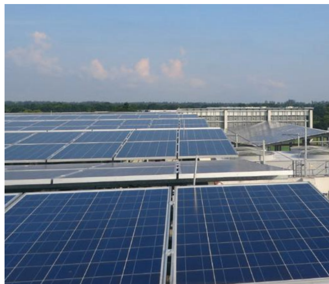
Keppel Land's corporate office at Bugis Junction Towers is fully powered by solar energy.
