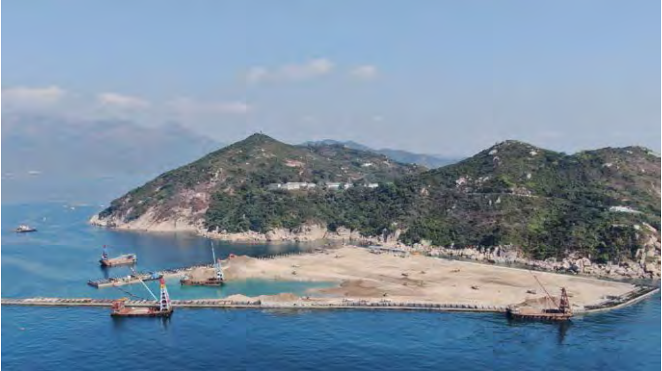
In 2020, significant progress was made on the land reclamation works for the HKIWMF.
