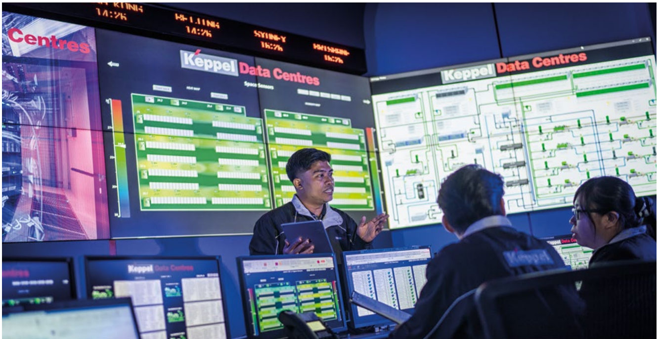
Keppel Data Centres is exploring artificial intelligence and machine learning technologies in daily operations and management, leveraging advanced sensor networks and big data analyses to perform predictive maintenance of its data centre infrastructure.
